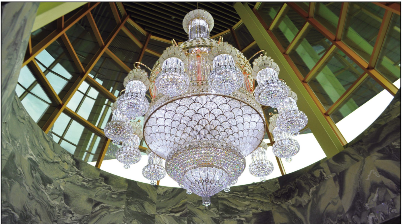
Korea GLAMI Company Lighting Project
